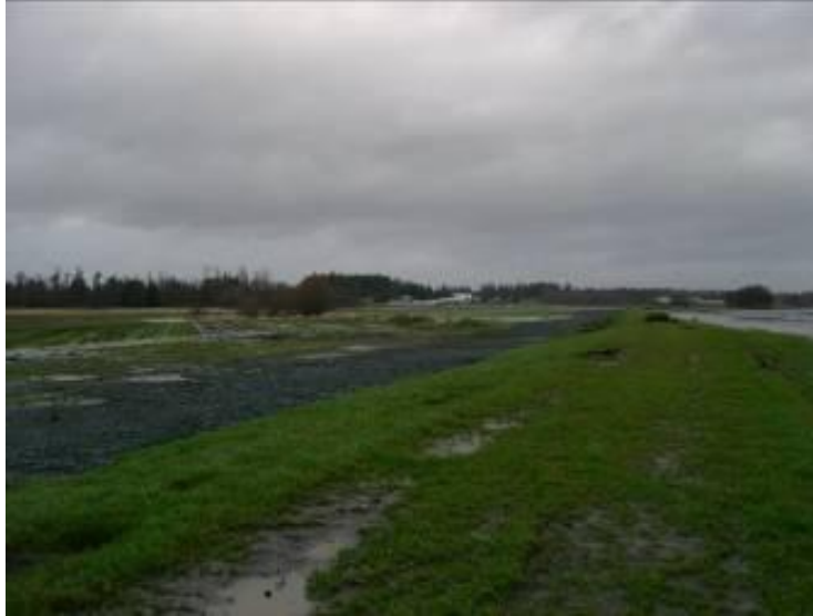
This shot, taken in December 2006, shows the good condition of the new Bertrand Creek dike shortly after the November flood. One of the protected farms lies to the left, with Bertrand Creek shown to the right.
