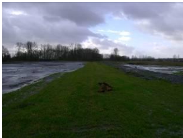
This is another shot of the newly completed dike. The farm is to the right and the area to be restored for salmon to the left. The Nooksack River lies beyond the line of trees in the distance.
